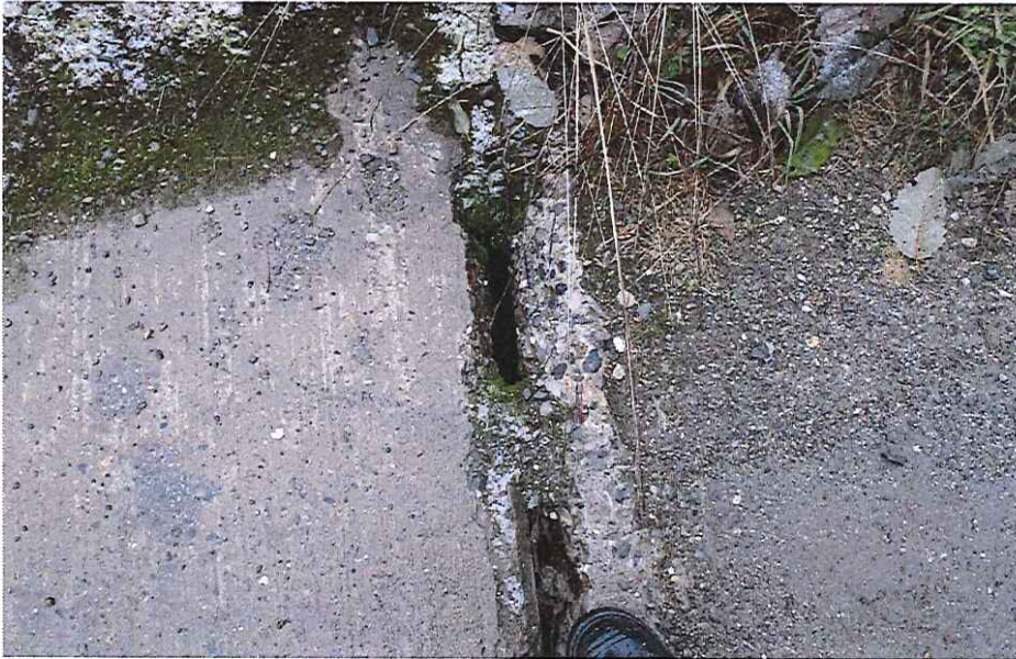
CK2018 Left ballast wall rebar exposed
